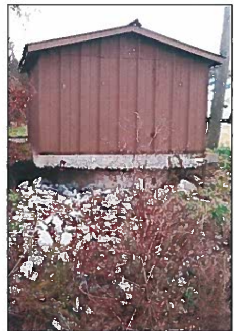
Campbell's Point Pump Station
