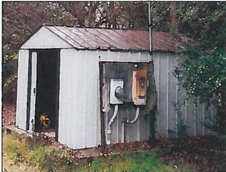
Yellowbrick Pump Station
