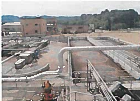
Renovated Digesters with Jet Aeration
