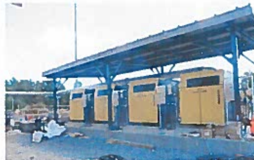
New Jet Aeration Blowers
