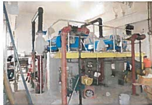
New Decanting Centrifuges
